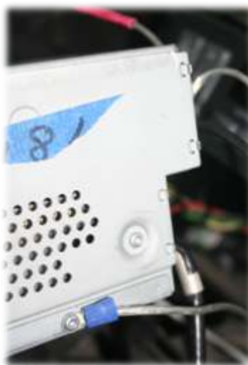
Image 7: Ring Terminals Used for Grounding
