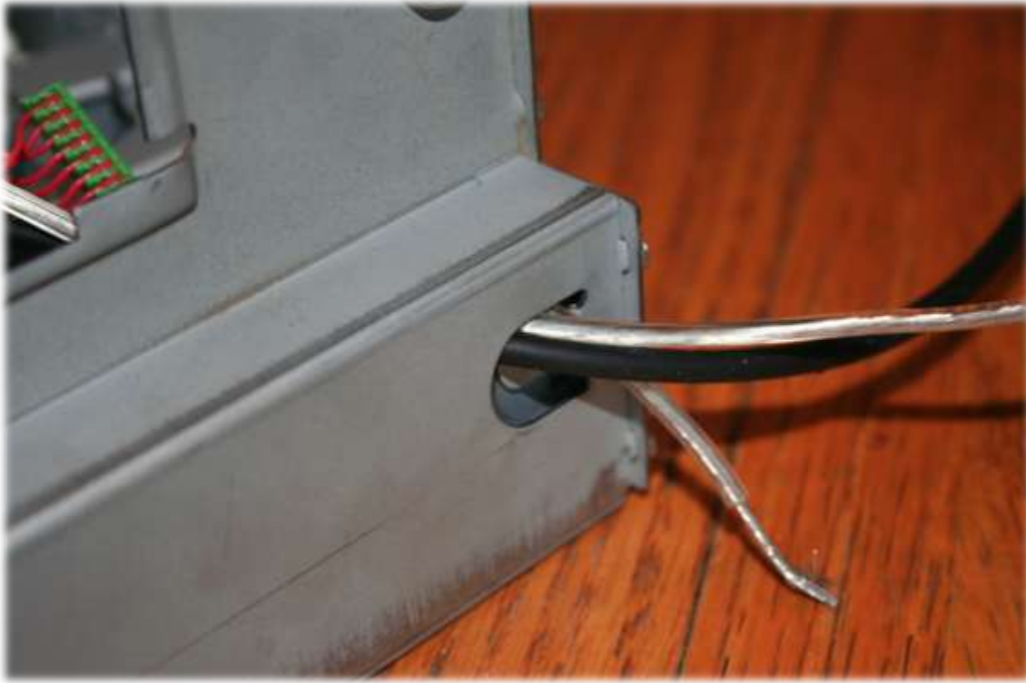
Image 5: Wires Routed Through A Hole
